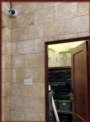
Figure 16: Storage Area with Cameras
