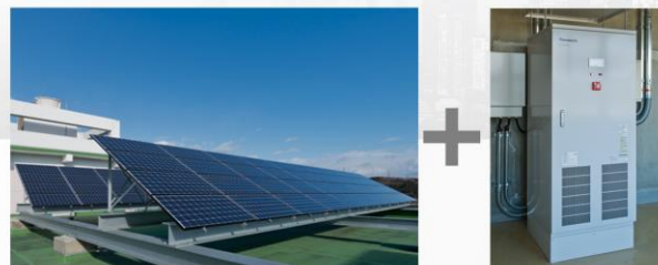
Solar power generation system
