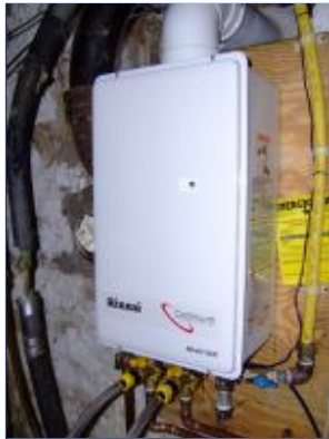
Rinnai tankless water heater warning code for lime deposits appears after 5 months
