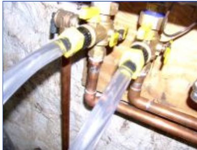
Valve drain caps removed, vinyl tubes with garden hose fittings screwed onto drain ports, water inlet/outlet valves closed, drain valves opened. Tube from transfer pump connected to cold water side, discharge from hot water side.
