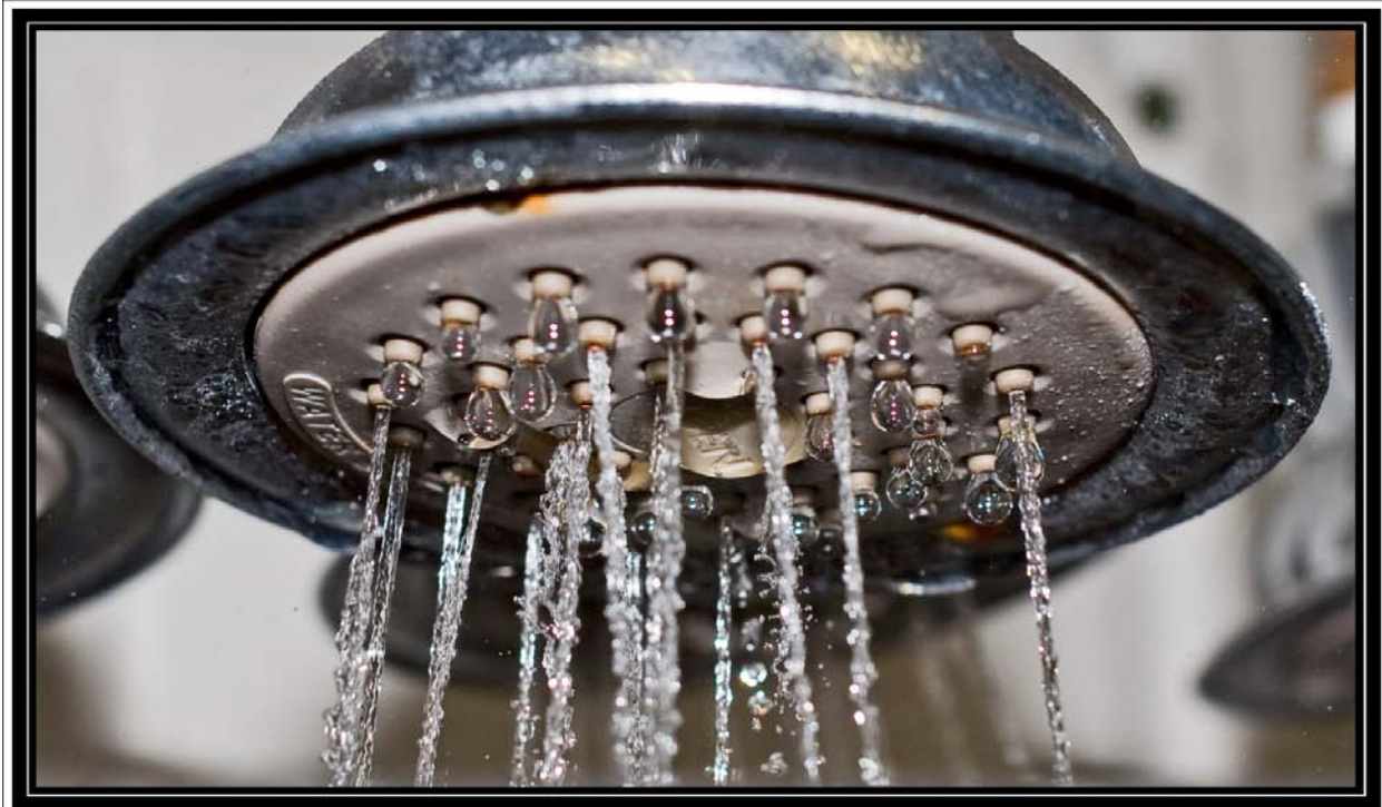
Figure 5-18. Typical spray pattern from one of the showerheads using unsoftened water at the end of the test.
