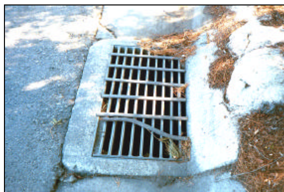
Retrofitted parallel bar grate, San Tomas Expwy
