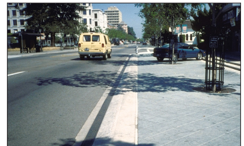
Slotted linear drain inlet, Castro Street, Mountain View.
