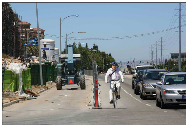
The bike lane and one travel lane on N. First Street were closed due to construction of condominiums, but space for bikes was preserved.
