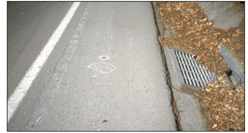
This drainage grate located off of the shoulder will not force cyclists into the travel lane in order to avoid it.
