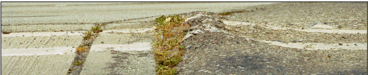
Asphalt bulge at end of bridge deck
