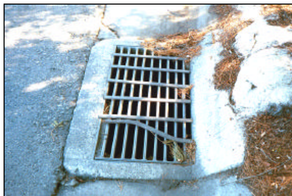
Retrofitted parallel bar grate, San Tomas Expwy
