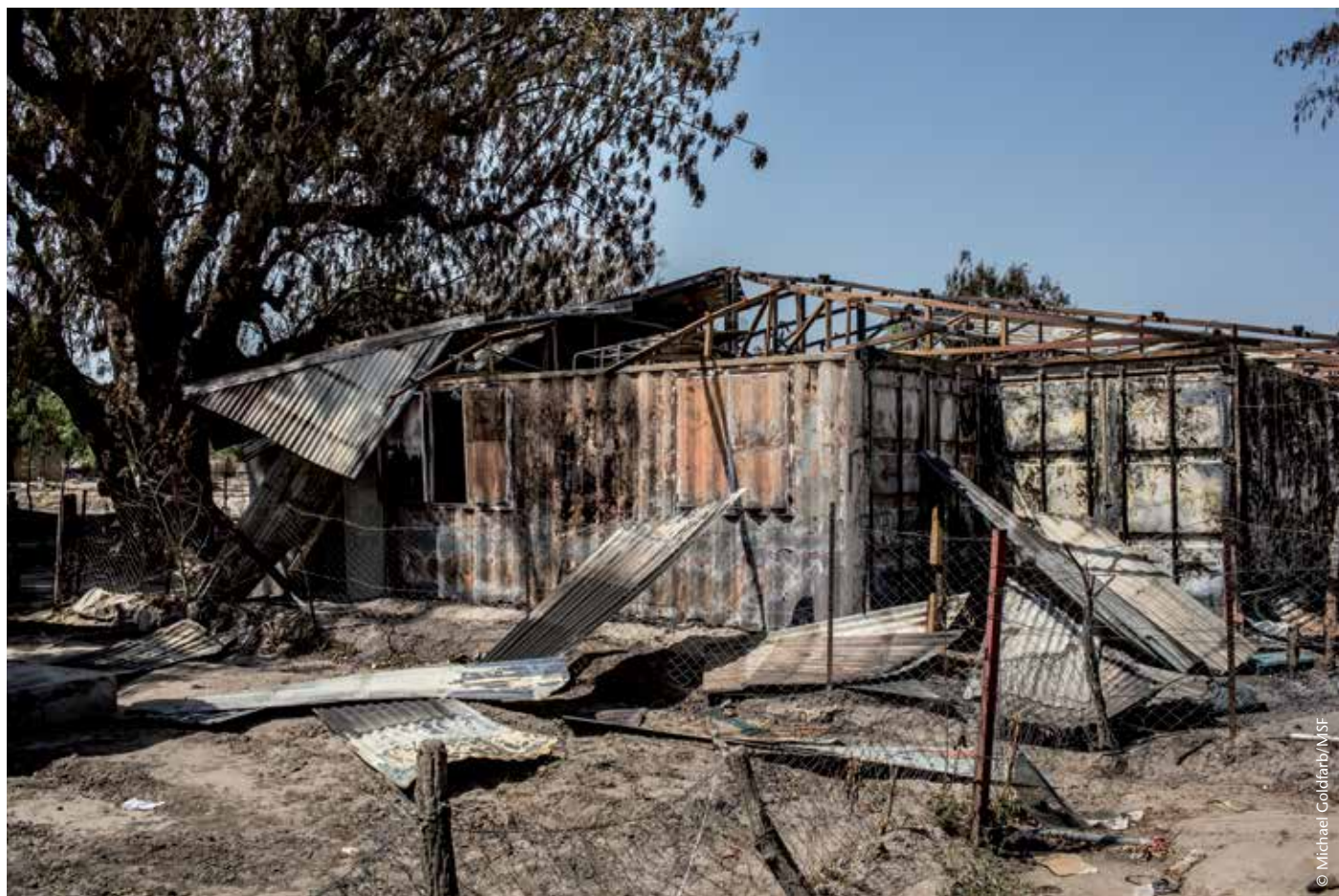
The hospital in Leer, South Sudan, after the building had been ransacked and set alight. It was the only specialist healthcare facility in Unity state.
