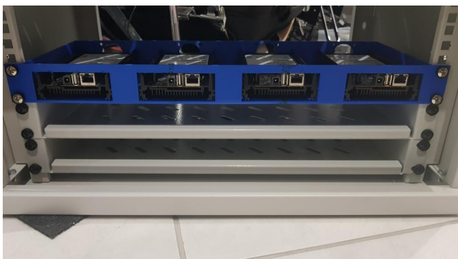
Figure 6 - The final rack setup looks like so:
