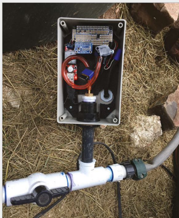
Above The whole thing is connected to the bottom of the tank in a small grey box
