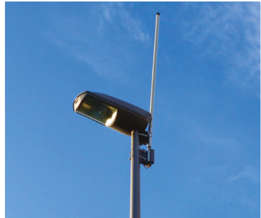
Above ♦ As part of Milton Keynes' smart meter project, LoRa gateways were mounted to lamp-posts across the city
