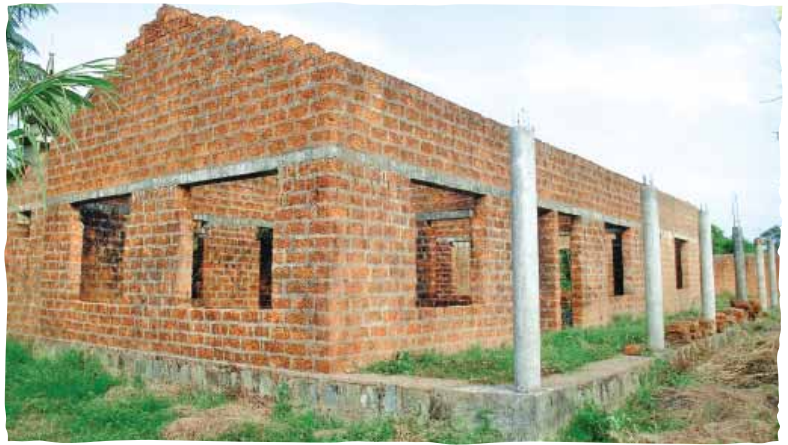
Hostel for SC / ST students sponsored by the Foundation under construction in Ankola, Karnataka
