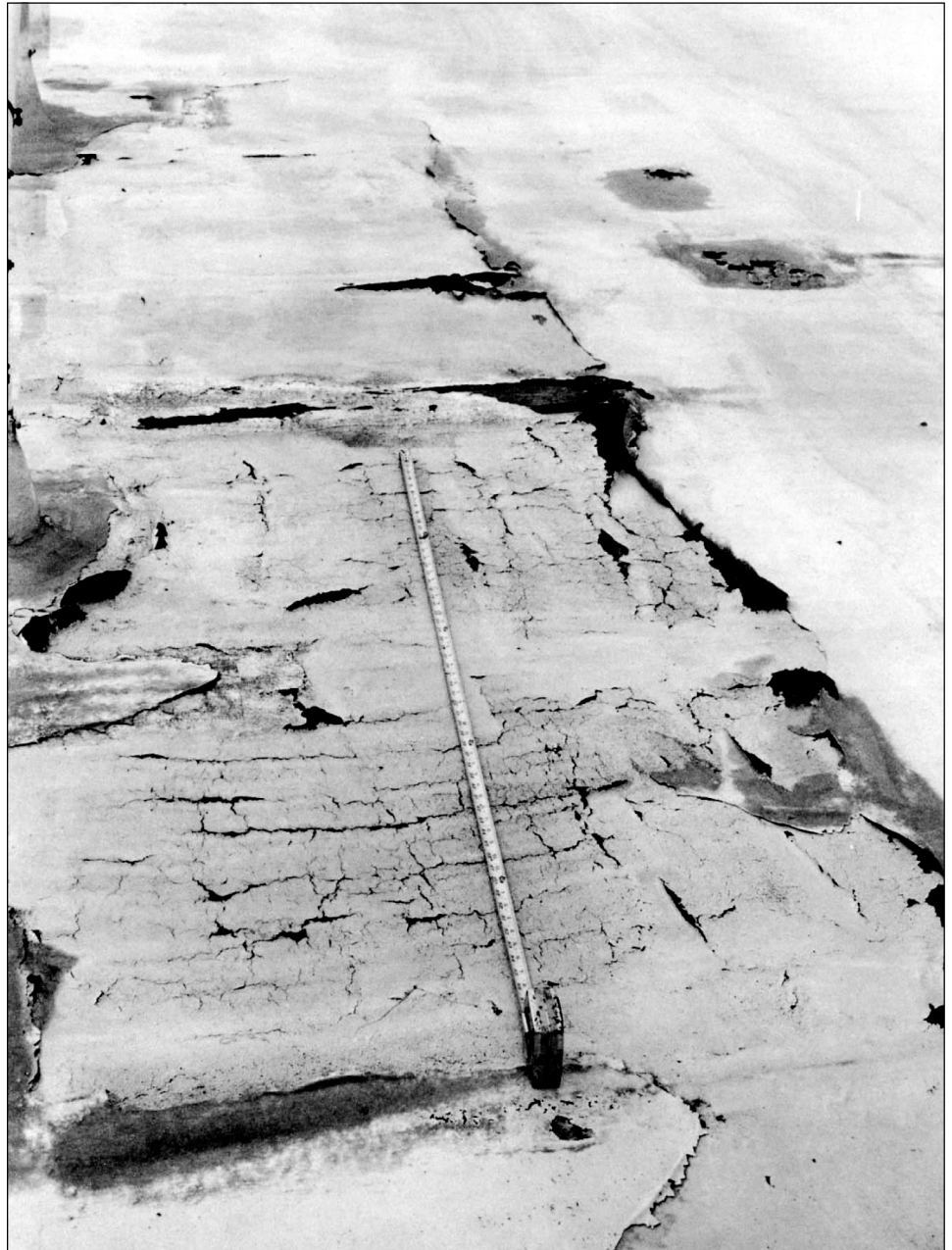
Figure 2: Roof Deterioration on the Vehicle Assembly Building at Kennedy Space Center (the tape shows a 5-foot section for perspective)
