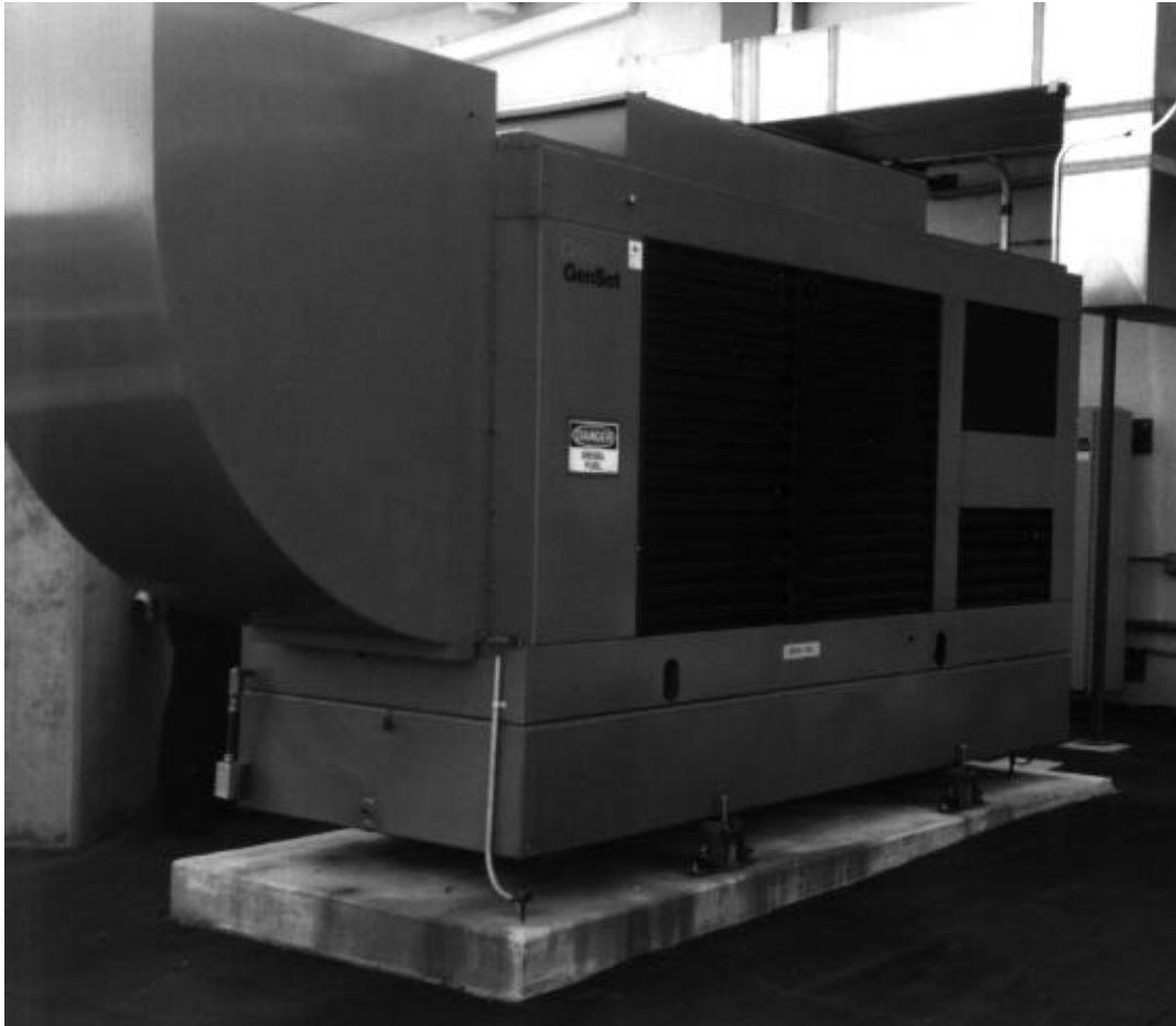
Figure 7. 375 BHP generator to be moved to March AFB outside of Building 2370
