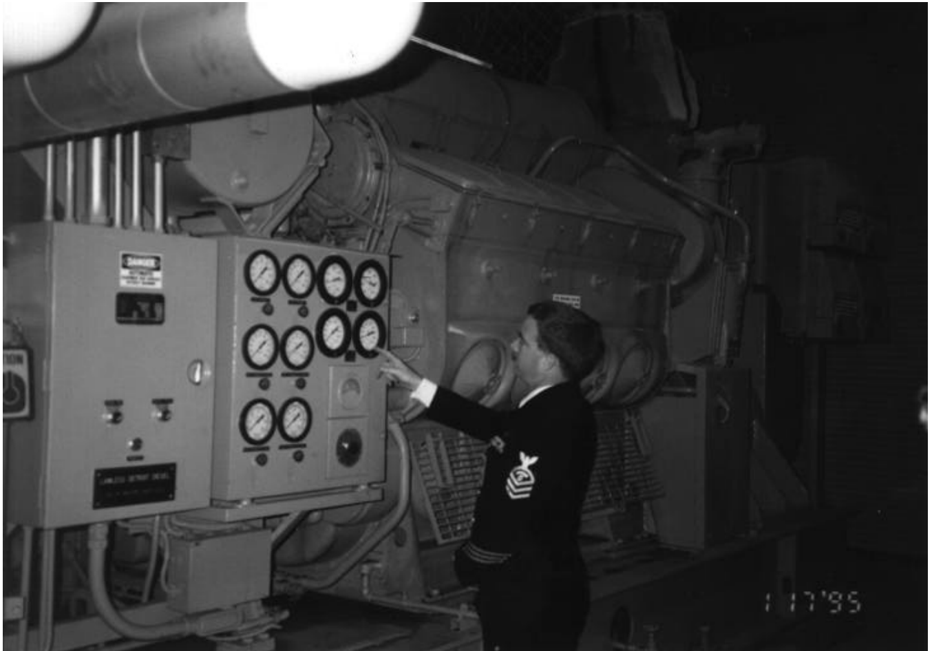
Figure 6. 1,200 BHP generator to be moved to March AFB outside of Building 2370
