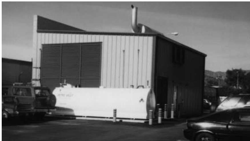
Figure 8. Fuel tank to be moved to March AFB outside of Building 2370. The building behind the tank houses the large generator at Sun Valley. A similar building will be built at March AFB.
