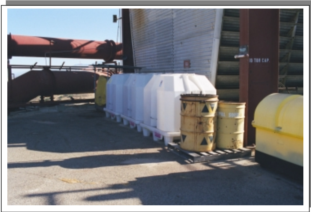
Non operating colling tower at HEPTS with asbestos containing panels.
