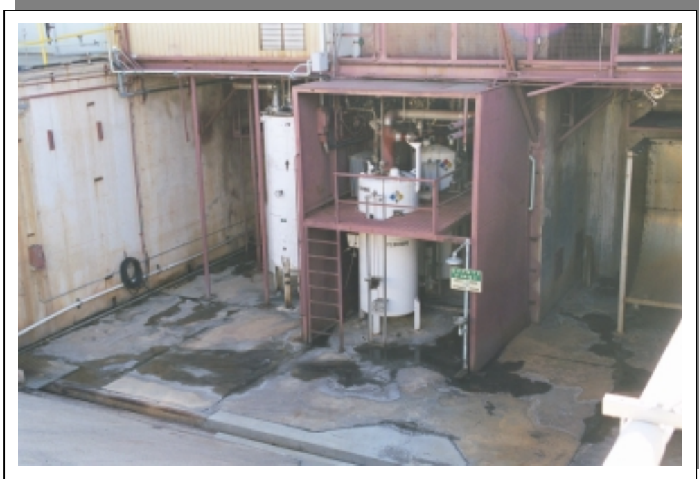
Fluorine Tanks at HEPTS.
