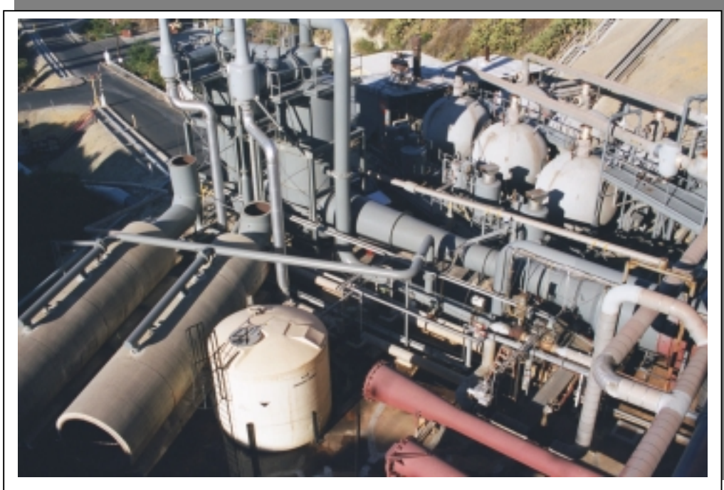
Steam plant and cooling water at VETS.
