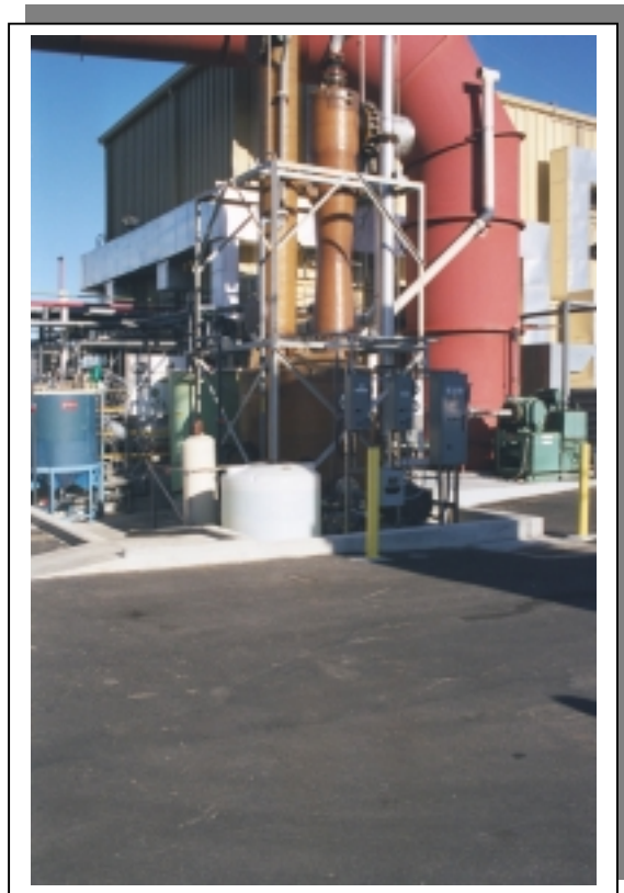
Scrubber at VETS
