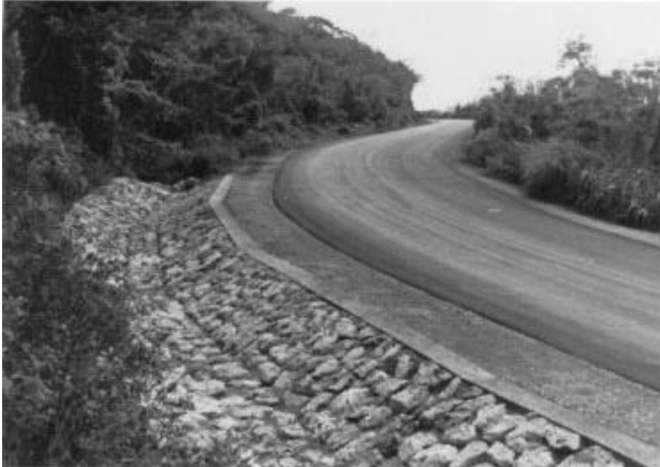
D.11 Looking South at Transition of Natural Swale to Riprap-lined Ditch Upgradient of Culvert I
