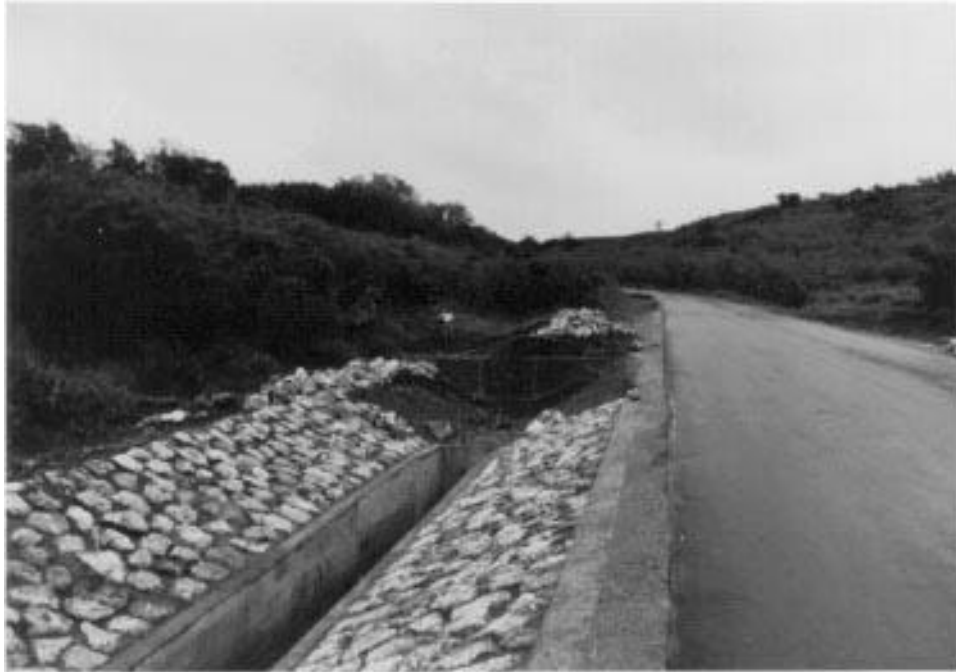
D.15 Looking East at Transition from Natural Swale to Riprap-lined Ditch at Outlet of Culvert IV
