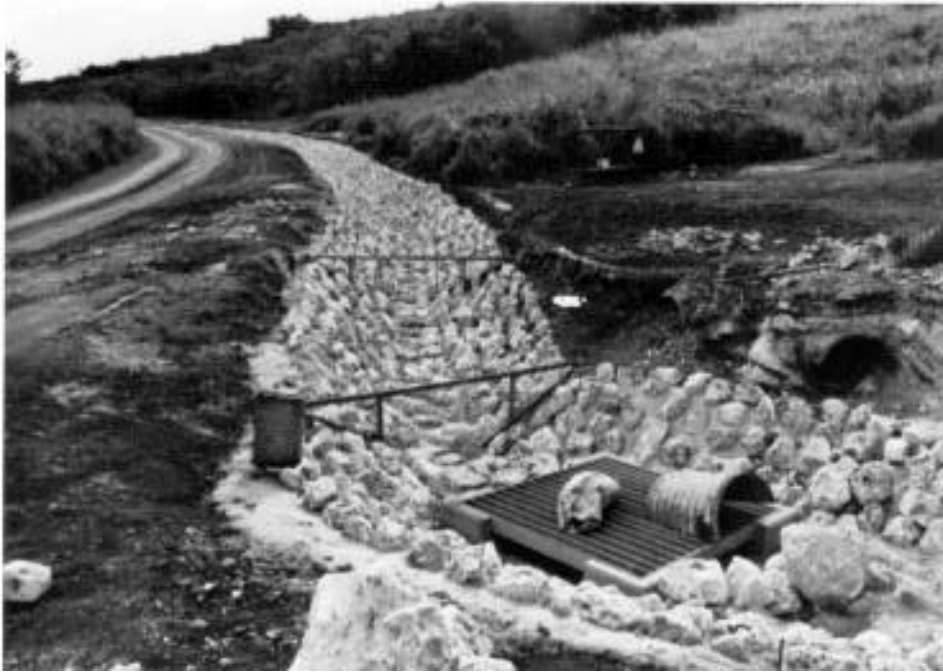
D.14 Looking Northeast into Inlet to Culvert III (work in progress at time of photo)
