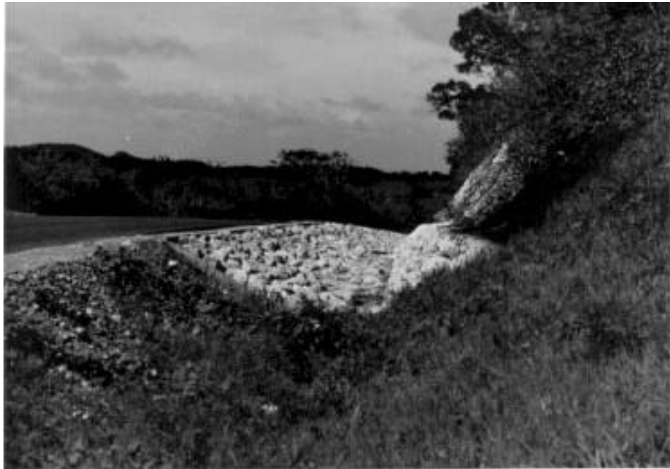
D.10 Looking North at Transition from Grass-lined Ditch to Riprap-lined Ditch Downgradient of World War II Bunker
