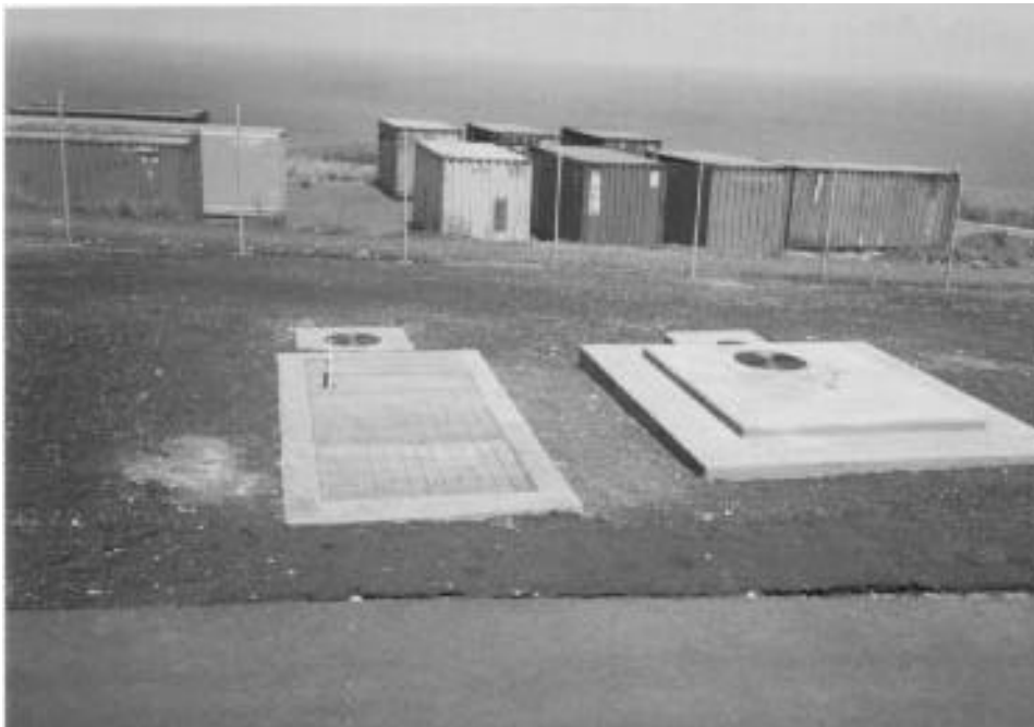
D.24 Oil-water Separator and Storage Tank at Radar Facility
