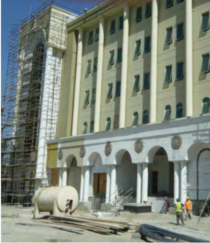
Ministry of Defense Headquarters Building under construction in Kabul, September 2014. (CSTC-A photo)
