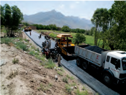
Sustaining non-security projects , like this DOD-funded road, could cost as much as 15% of Afghanistan’s GDP. See Special Project 14-72-SP. (ISAF photo)
