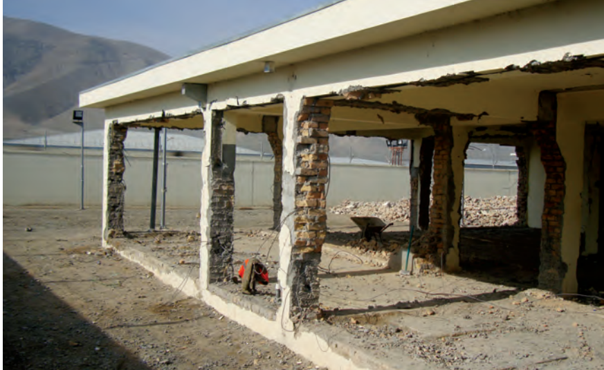
Building 17 , one of the three most seriously damaged structures at Baghlan Prison, was demolished due to safety concerns. See Inspection Report 14-62-IP. (INL photo)
