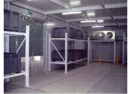
The cold-storage facility at Gereshk includes shelving and cooling equipment. See Inspection Report 14-82-IP. (RC-SW photo)
