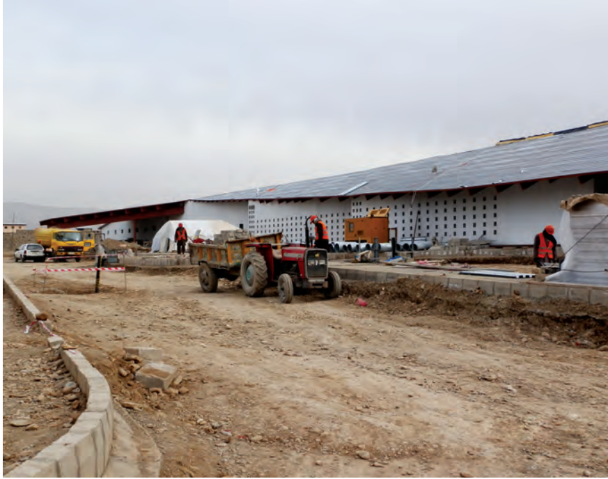
The Gardez hospital , shown here under construction, has annual operations and maintenance costs that are too high to be sustained by the Afghan government. See Inspection Report 14-6-IP and Audit Report 13-9. (SIGAR photo by Lise Pederson)
