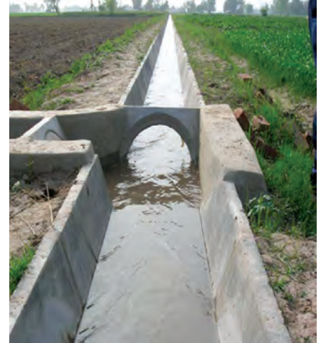
Cement irrigation canals installed by USAID Afghanistan as part of an agriculture project. (USAID photo)
