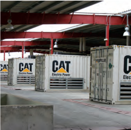
Diesel generators are used to provide electricity until NEPS and SEPS can be expanded and connected. (SIGAR photo by Steven Mocsary)
