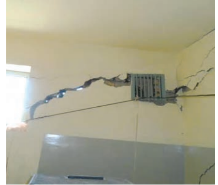
Soil settlement led to serious structural damage to, and eventual demolition of, building 17 at Baghlan Prison. (State Department photo)
