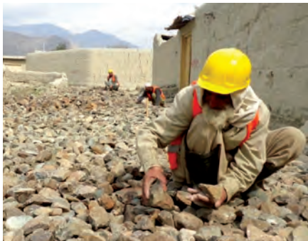
The Khani Baba street network repair project aims to rehabilitate 800 meters of village streets and drainage trenches to build confidence in the local government. (CCI photo)
