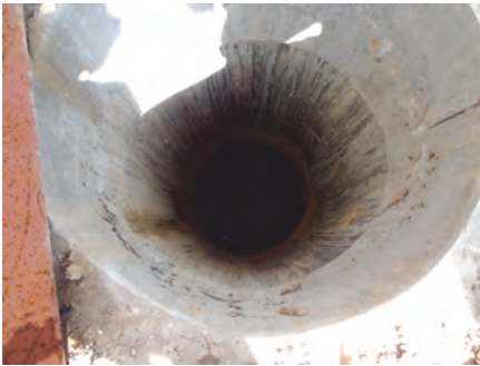
Neither access point to the septic tank has a solid cast iron cover or a permanent ladder, both of which are required by the contract. (SIGAR photo by Ron Riach)
