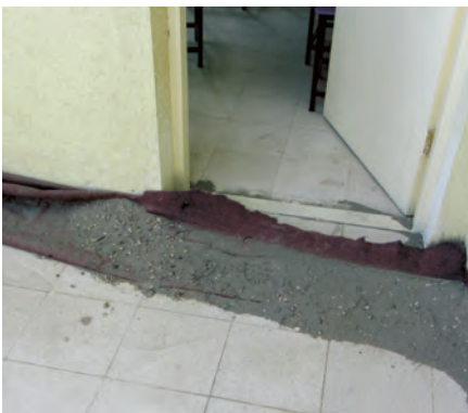
SIGAR auditors discovered a second floor terrace that slopes toward the classroom door, requiring an improvised dam to stop rainwater from flowing into the classroom. (SIGAR photo by Les Thompson)
