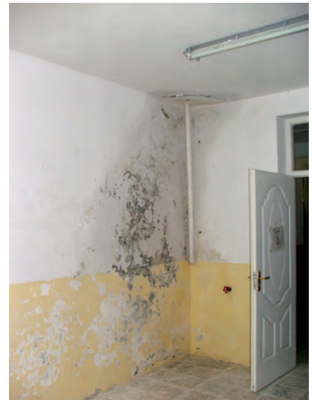
A leaky roof at the Salang Hospital led to mold and mildew on the ceilings and walls. (SIGAR photo by Brian Flynn)
