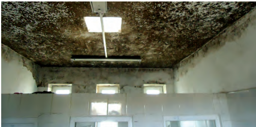
Archi District Police Headquarters has hazardous mold on walls and ceilings of living/working facilities for about 40 ANP personnel. (SIGAR photo)
