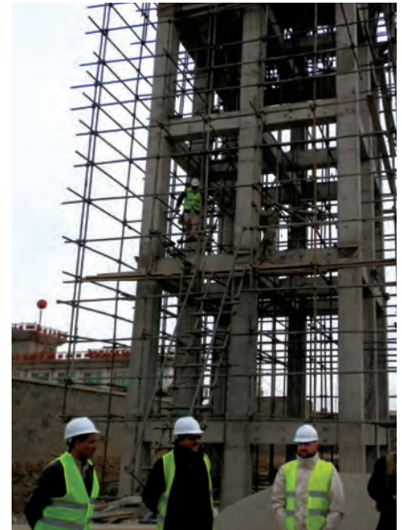
SIGAR inspectors examine the construction still in progress at Gardez Hospital. (SIGAR photo)
