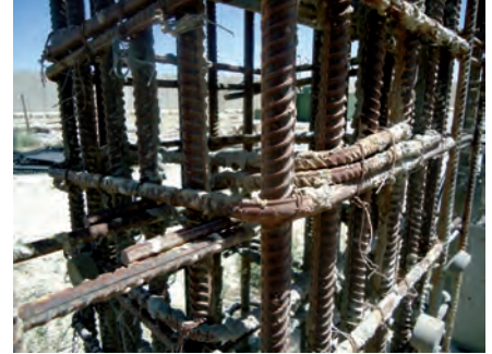
Failure risk at Parwan Justice Center: rebar bound with wire instead of being welded. (SIGAR photo)
