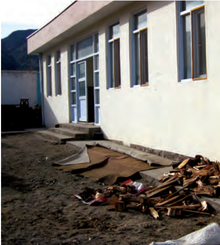
At Walayatti Medical Clinic, no structures were built to specifications, or are occupied. (SIGAR photo)
