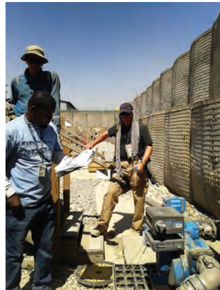
Checking fuel-pump meters against delivery records helps detect and deter fuel theft, a multi-million-dollar problem in Afghanistan. (SIGAR photo)
