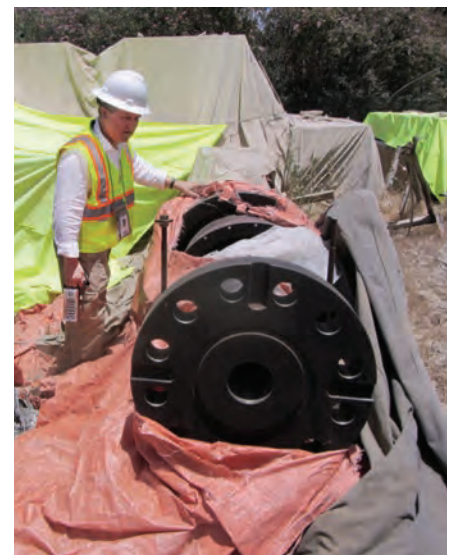
Parts for the third turbine at the Kajaki Dam power plant have languished outdoors under tarps for years, awaiting installation. (SIGAR photo)
