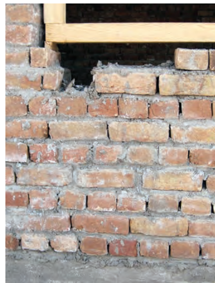
Construction deficiencies found at Bathkhak school include large gaps between bricks in the wall that support the ceiling and roof. (SIGAR photo)
