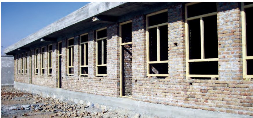
A school in Bathkhak province , built with wood windows and brick walls instead of the more durable vinyl and stronger cinderblock required by contract. (SIGAR photo)
