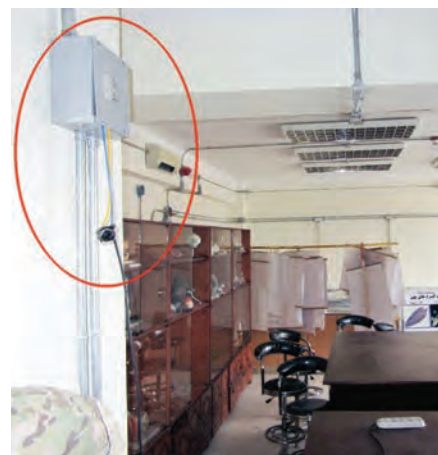
Improper electrical wiring and overloaded electrical circuits (circled in red) demonstrate the risk of fire and electrical shock to Sheberghan school occupants. (SIGAR photo)
