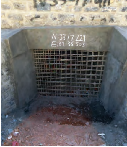
Culvert-denial systems like this grid of steel rods prevent insurgents from easily placing explosives beneath roads. (SIGAR photo)
