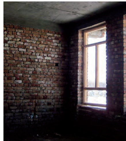
A risk of collapse exists at the Bathkhak School because the contractor installed a concrete-slab roof atop brick walls instead of the wood-framed roof atop concrete blocks as required by contract. (SIGAR photo)
