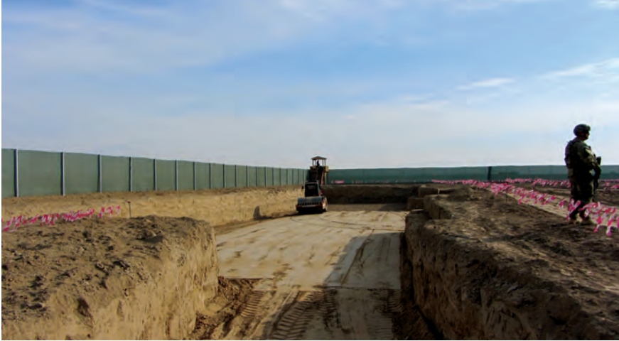
A U.S. soldier provides security at the construction site of the ANP Main Road Security Company compound. (SIGAR photo)
