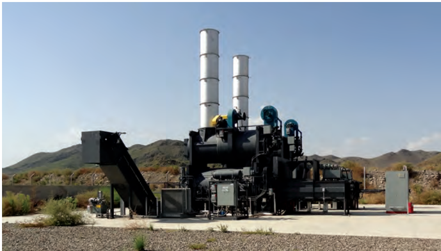
Solid waste incinerators constructed at FOB Salerno. (SIGAR photo)
