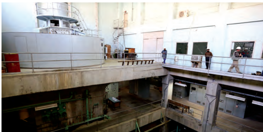
The turbine hall at the Kajaki hydroelectric station in Helmand Province currently has two turbines like the one visible at left. U.S. aid will provide for installation of a much-needed third turbine delivered in 2008. (State Department photo)
