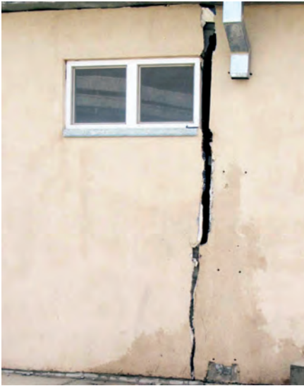
Failure to properly stabilize soil before constructing the Camp Pamir ANA garrison in Kunduz Province led to serious structural damage from soil settling, such as to this building. (SIGAR photo)
