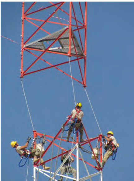
A U.S. Air Force crew at Bagram Airfield connects sections of a 170-foot communications tower to expand radio-communication range. (U.S. Air Force photo)
