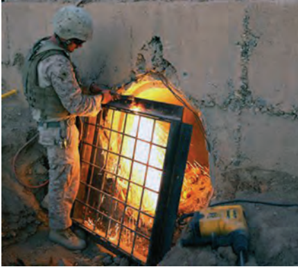
A U.S. Marine installs a culvert denial system in Afghanistan. (DoD photo)
