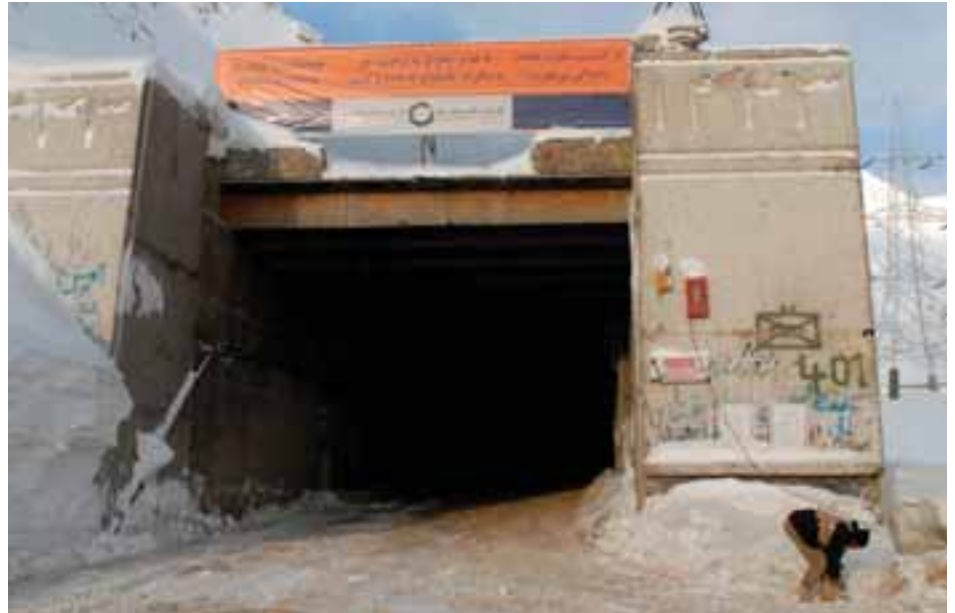
Repair work resumes on the Salang Tunnel in the Hindu Kush mountain range, the only year-round link between northern Afghanistan and Kabul. The project, which is conducted by the Ministry of Public Works and USAID, will ensure that 7,000 vehicles can continue to use the tunnel each day. (CJTF-101 photo, SGT Scott Davis)
