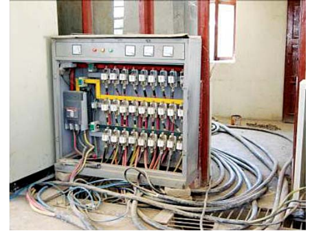
A 400-kV distribution panel as rewired by Afghan plant operators at Khowst Power Plant 1. (SIGAR photo)
