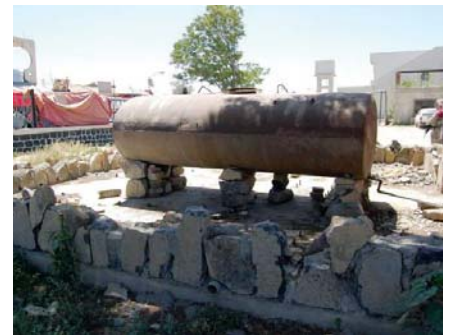
A rusted fuel tank resting on rocks is used as the fuel reservoir for Khowst City Power Plant 2 instead of the two new 6,000-liter fuel tanks that should have been installed in accordance with the project design. (SIGAR photo)
