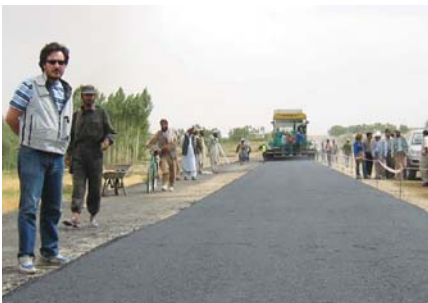
Pavement is laid on the Kabul-Kandahar Road, part of the Ring Road. (USAID photo)
