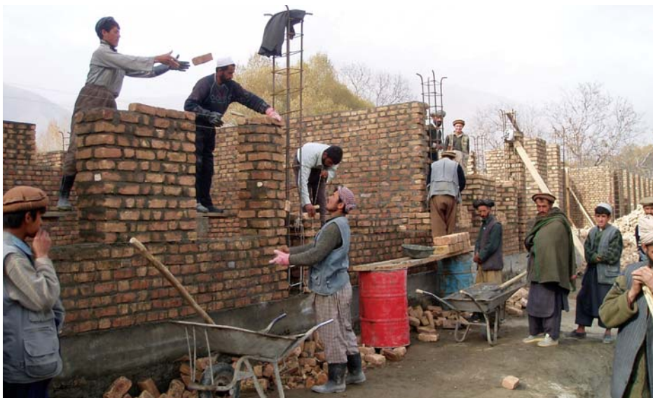
The construction of Jurm School, a USAID-funded school construction project, has created jobs for Afghan men. (USAID photo, Ben Barber)
