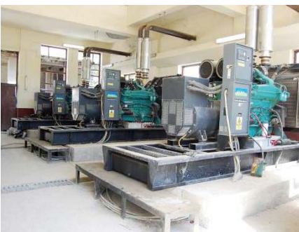
The three new 500-kW generators at the Khowst Power Plant as they appeared during the SIGAR inspection visit on May 16, 2009. Of these three new generators, only two are operational; the third is awaiting replacement parts. (SIGAR photo)
