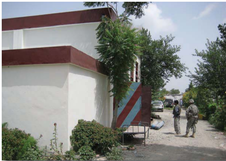
Khowsat power plant following the installation of new generators and power distributors in June 2008
