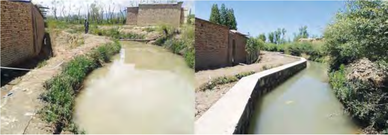
Before and after photographs of a flood protection wall built by USAID in Ahmadabad District, Paktiya Province. (USAID photo)
