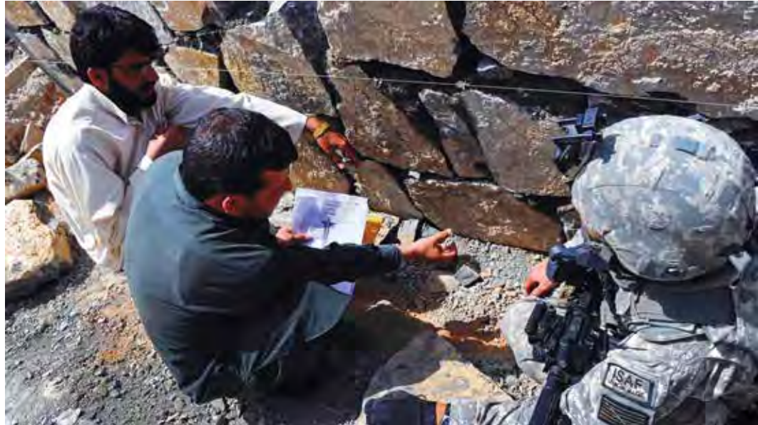
U.S. Navy Lt. Jg. Anthony Delgadillo, Khost Provincial Reconstruction Team engineer, looks at the foundation for an addition to the Sadiq Rohee boys' school with the site engineer, on June 10, 2010. (U.S. Air Force photo by Sr. Amn. Julianne M. Showalter, Khost PRT public affairs office)
