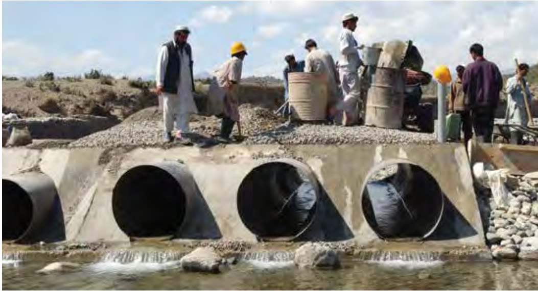
Afghan laborers build a new CERP-funded aqueduct system in Khost Province on September 23, 2006. (Photo by S. Sgt. Robert R. Ramon, 345th Mobile Public Affairs Detachment)
