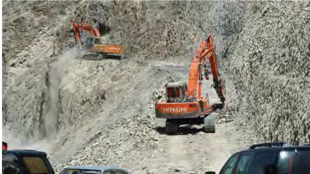
USAID road construction efforts along the Khost-Gardez road in March 2010. (USAID photo)
