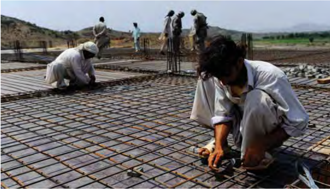
Members of Khost Provincial Reconstruction Team check the quality of the work done on the Hassan Khot school roof on July 3, 2010. (Photo by U.S. Air Force Sr. Amn. Julianne M. Showalter, Khost Provincial Reconstruction Team Public Affairs Office)
