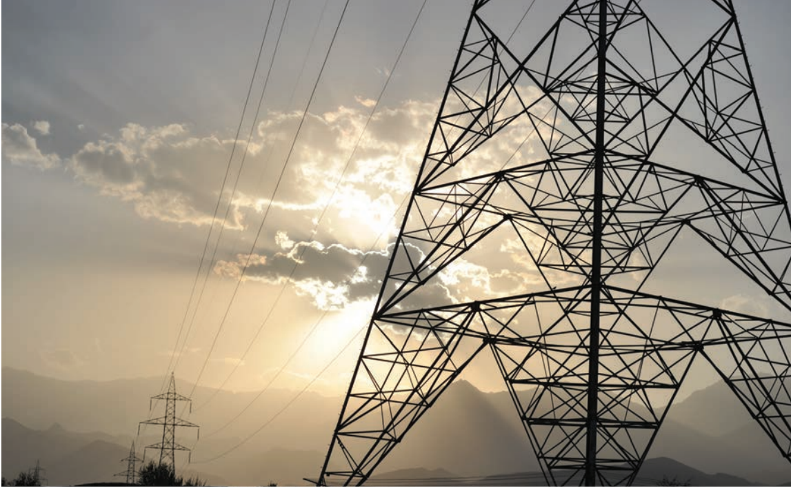
Towers erected in a transmission-and-distribution improvement project carry power on the outskirts of Kabul. (Asian Development Bank photo)
