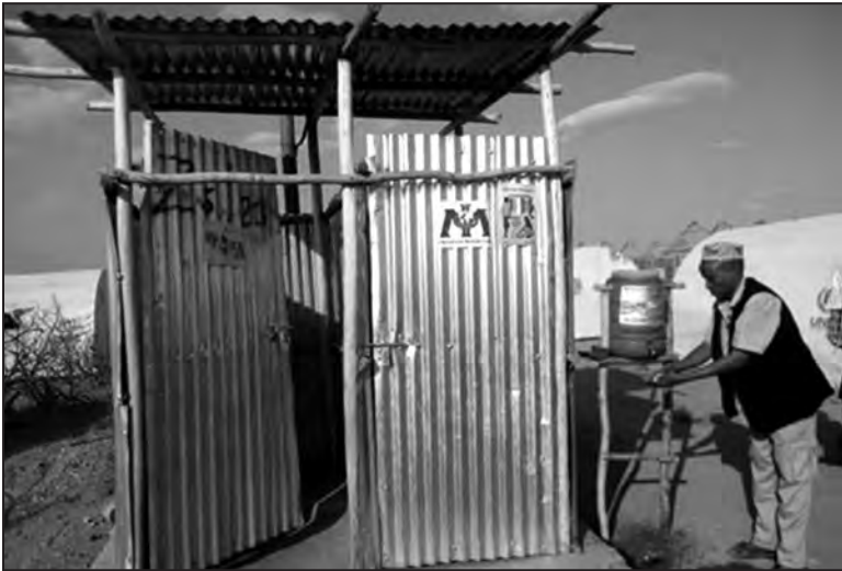
Figure 1-2. A man washes his hands in a Kobe refugee camp. 10 This latrine and water source are shared by four families. A weaponized DPRE attack on vulnerable resources can cause widespread contamination before proper identification of the threat. Photo source: Negash, Meron Tsehaye. “Sanitation & Hygiene Efforts in Kobe Refugee Camp: Mohammed’s Story.”
