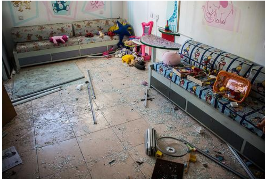
Above: A rocket from the Gaza Strip severely damaged a children’s health clinic in Ashkelon, July 16, 2014. (Source: IDF)
