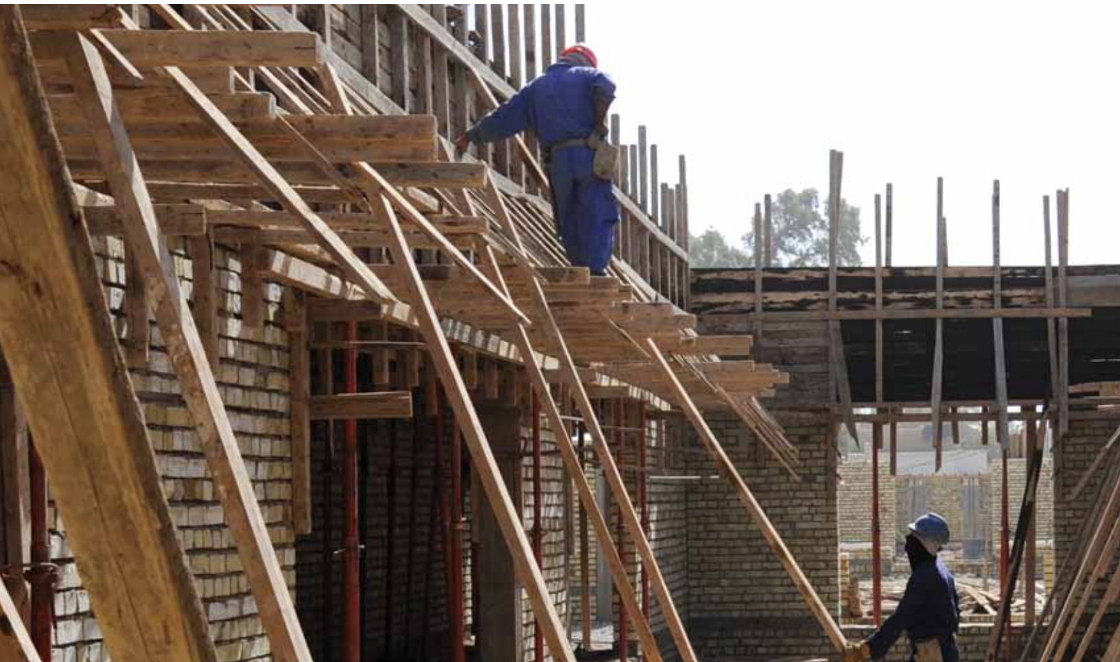
Iraqi contractors on school construction site, Baghdad, Iraq. (U.S Air Force photo)
