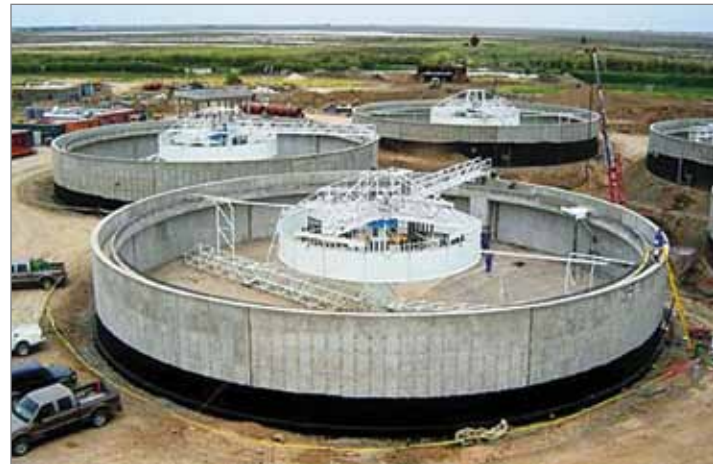
The Nassiriya water-treatment plant, Iraq, 2007. (U.S. Army Corps of Engineers photo)
