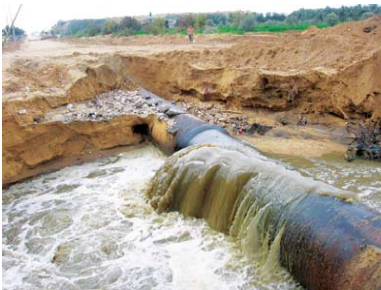
Figure 5. Beit Hanoun Wastewater Pressure Line on 21-1-2009 3
