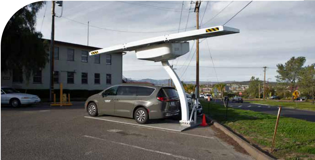
An electric van docks at a new solar-powered electric vehicle charging station on Marine Corps Base Camp Pendleton, CA. The self-contained, portable charging stations are independent from the electric grid, can be installed immediately, fit over a parking spot, and be moved to support mission essential tasks or be used during emergencies as a power bank, increasing overall mission resilience for U.S. forces. The Marine Corps' Southwest Region Fleet Transportation Office recently acquired two of these charging stations to add to their existing permanent electric vehicle charging infrastructure at Camp Pendleton, Jan. 12, 2022.
