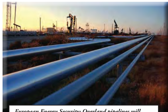
European Energy Security: Overland pipelines will continue to be an economic and political driver across European Command's area of focus.
