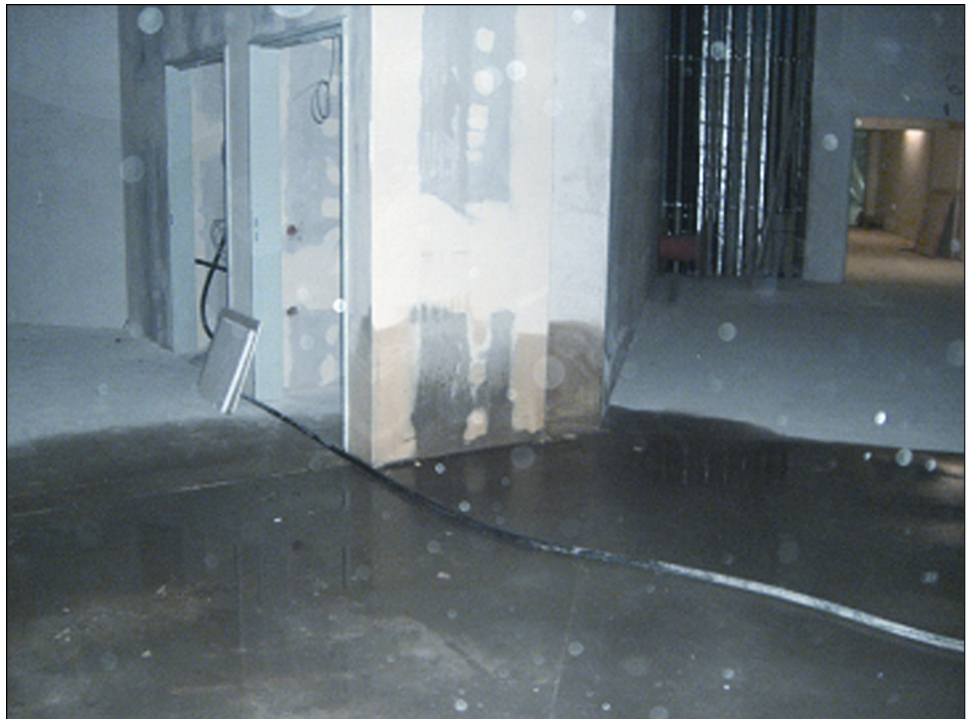
Figure 2: KMCC Damage from Leaks in Roof
