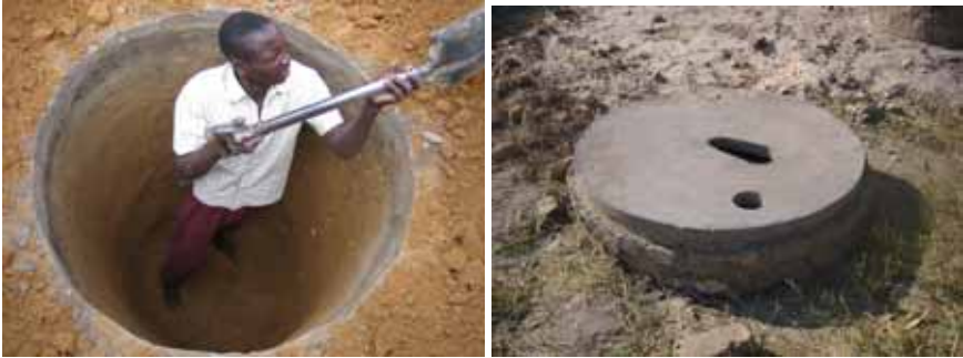
First pit being dug down to 1.5m depth. The concrete slab is then fitted and sealed with weak cement mortar.
