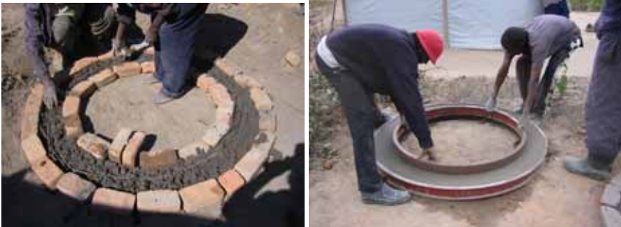
Concrete ring beams can be cast inside a brick mould or within specially made steel moulds. In this case the ring beam has an ID of 1m.
