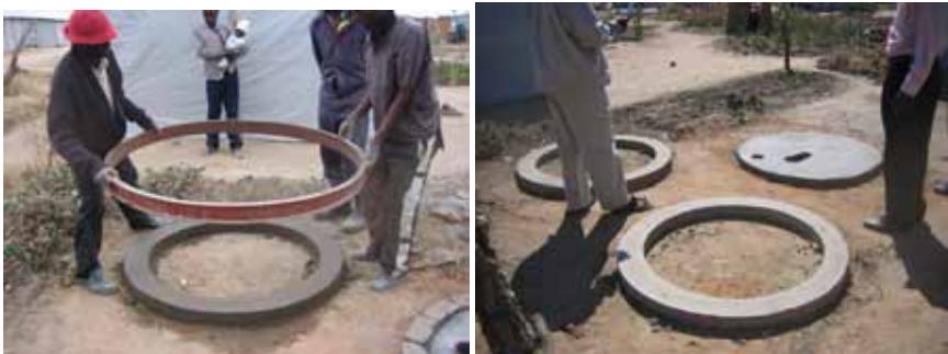
Steel ring beam shuttering in use. Two ring beams are cast and a slab
