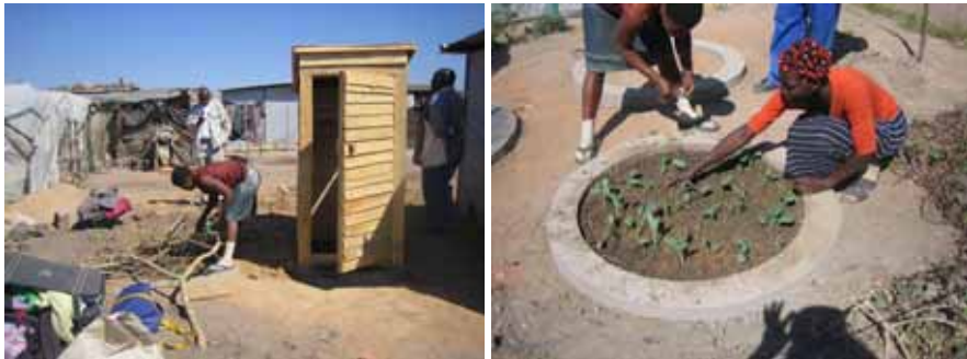
A suitable superstructure is then mounted on the slab and the toilet can be put to use. The soil within the second ring beam is planted with suitable vegetables and kept watered.
