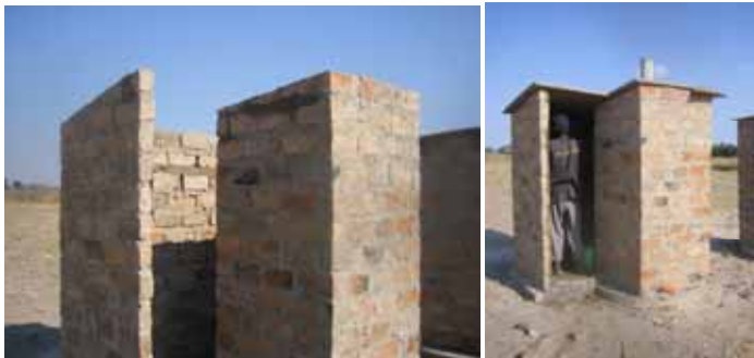
The walls are built up and roofing panels added. A short length of tubular pipe is mounted through the roof on a concrete plate (see detail elsewhere)
