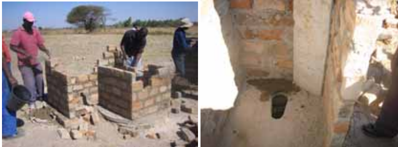
Brick walls are built up. In this case the pipe is made of a concrete panel mounted on interior wall over vent hole.
