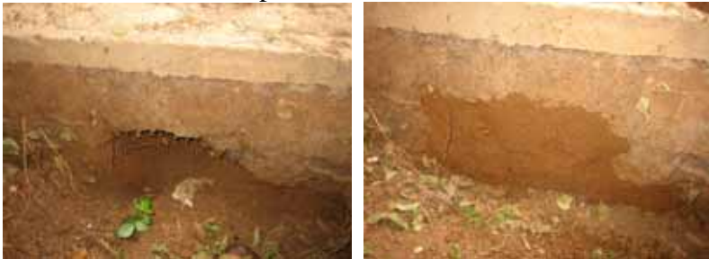
Photos showing eroded section of pit wall under ring beam. This has been filled with a mix of red soil and cement to stabilise.
