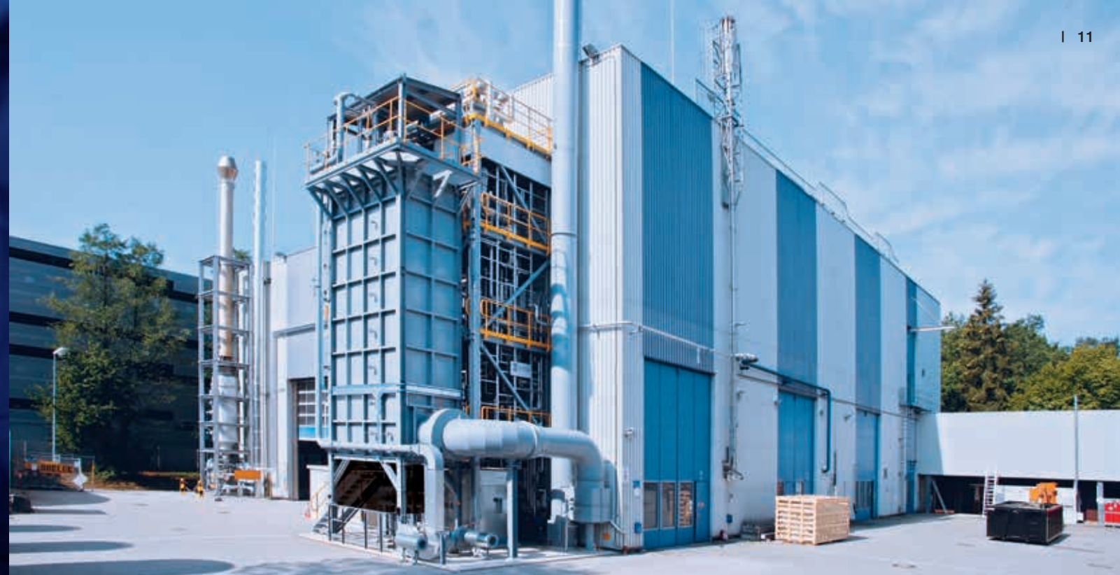
Reformer in Pullach
