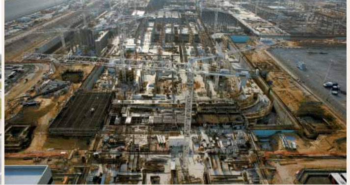
Construction of a new terminal and concourses at Dubai International Airport is on schedule.
