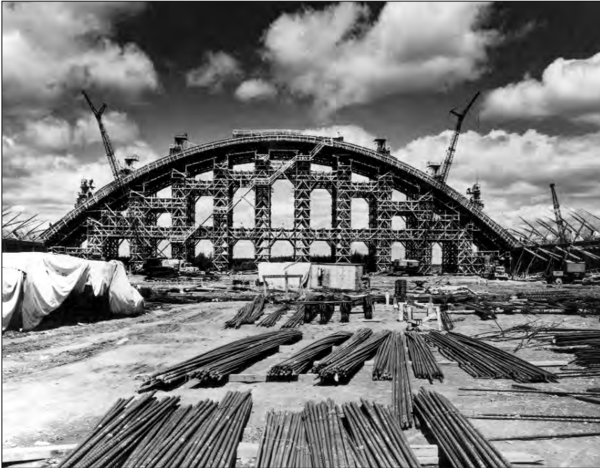
A B-36 hangar under construction in 1948 at Limestone (later, Loring) Air Force Base, Maine, the first new Strategic Air Command base.
