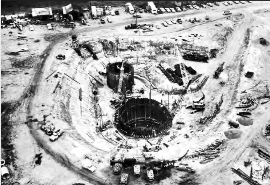
Construction site, early 1960s, for the Series F Atlas ICBM “silo-lift” launcher at Plattsburgh Air Force Base, New York. On a “silo-lift” launcher, the missile is stored vertically within a hardened, underground silo.
