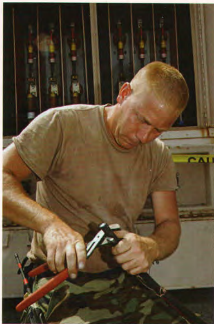
9/12/2005, TSgt Jody Saatoff from the 119 th Civil Engineer Squadron, North Dakota ANG, works on power cables that will supply electrical power to various personnel tents erected at Gulfport CRTC, MS. (Photograph by SMSgt. David Lipp, 119 th Fighter Wing, North Dakota ANG)
