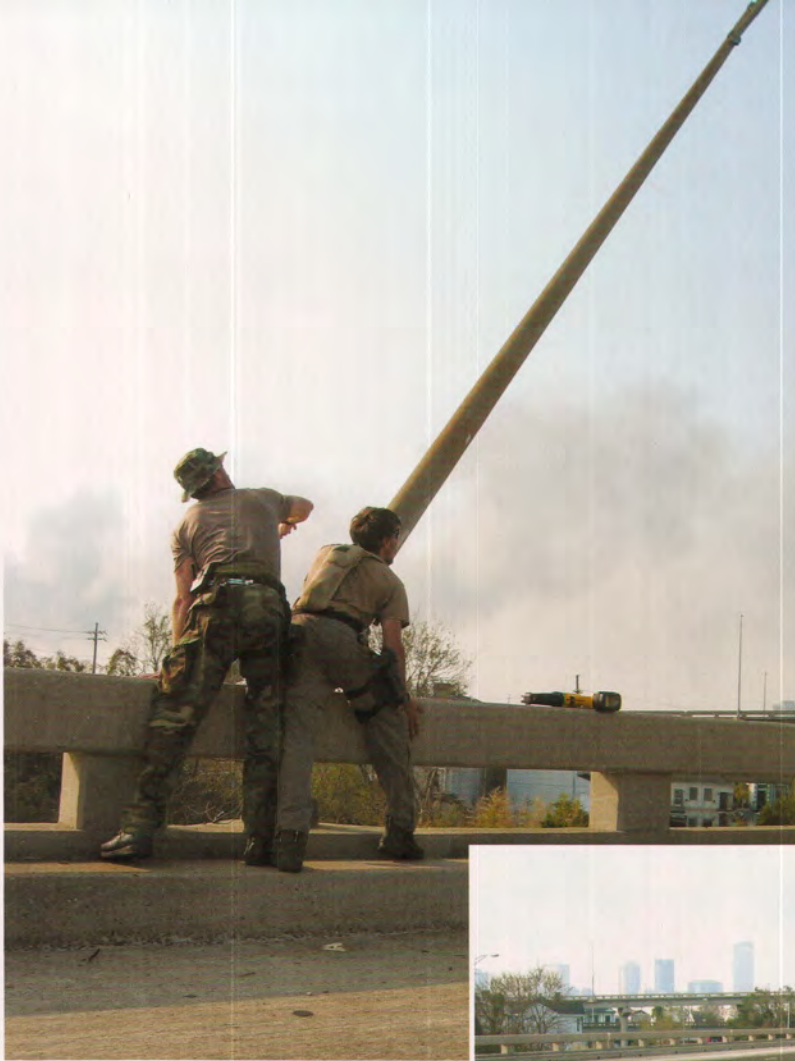
ANG combat controllers cutting down light poles along I-10. (123rd STS Photograph)
