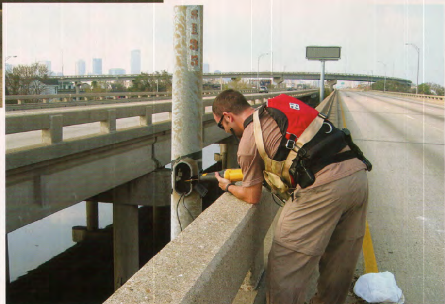
An Air Guard combat controller prepares to bring down another light pole along I-10. (123 rd STS Photograph)
