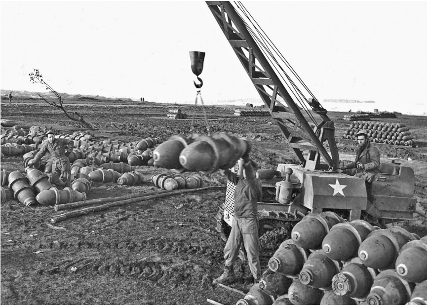
Supplying the Air Campaign in Southern France. Armorers at a hastily constructed airfield in southern France use a crane to stack 500-pound general purpose bombs. The establishment of facilities such as this one allowed XII Tactical Air Command to provide steady air cover for 6th Army Group's advance during the autumn of 1944. National Archives.
