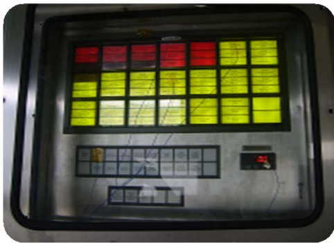
Temperature Measurement And Alarm Test
