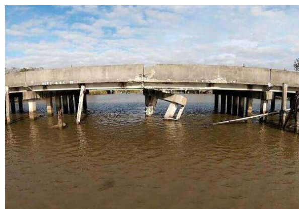
Figure 59: Bayou Ramous Bridge Strike
