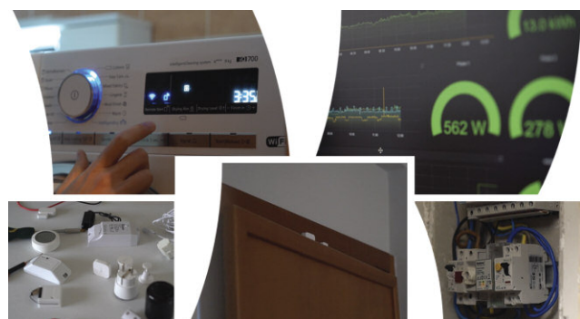
Figure 1: Integration of IoT and smart grid technologies in residential settings. Hardware components including smart appliances, IoT sensors and smart meters installed within the electrical panels.
