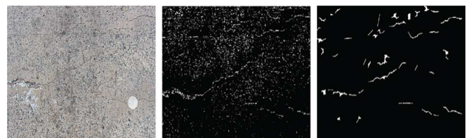
Fig. 3. (Left) Original image showing a surface with cracks. (Center) Image showing the output of a prior crack detection algorithm [15]. (Right) Image showing the output of our algorithm.
