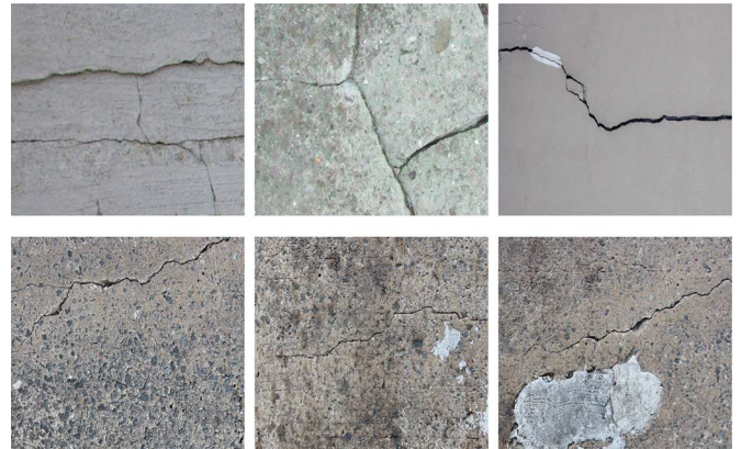
Fig. 2. (Top Row) Prior work uses images that are high contrast and low clutter similar to the images shown. Simple methods such as edge detection and thresholding for binarization can be applied for these images. (Bottom Row) Real bridge deck images from our work shows significantly more distractors and pose a more challenging crack detection problem.
