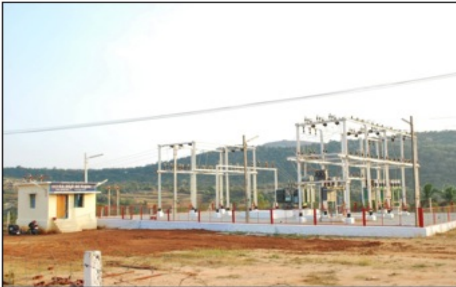
5 MVA Common Substation
