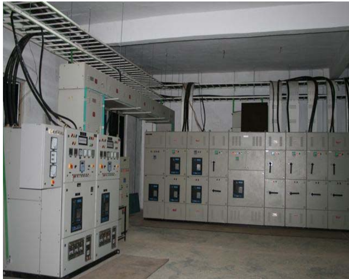
Electrical Panel Room
