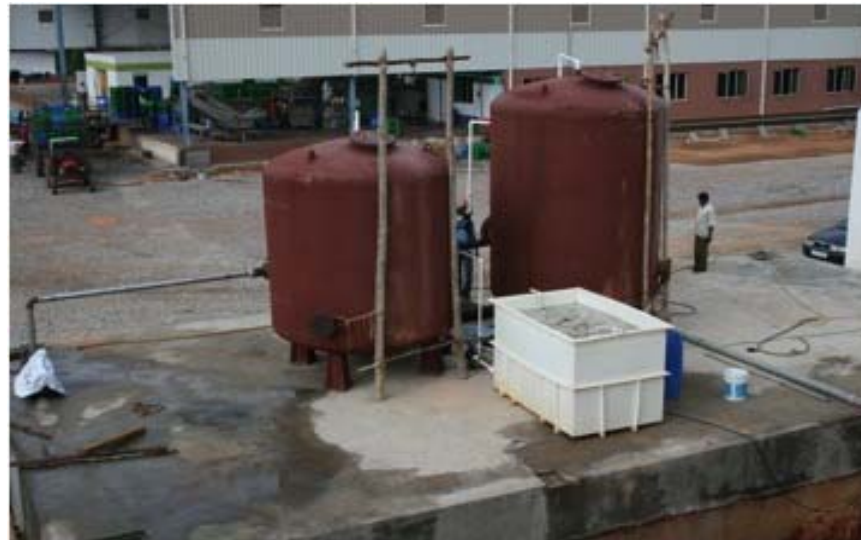
Central Water Softener Plant
