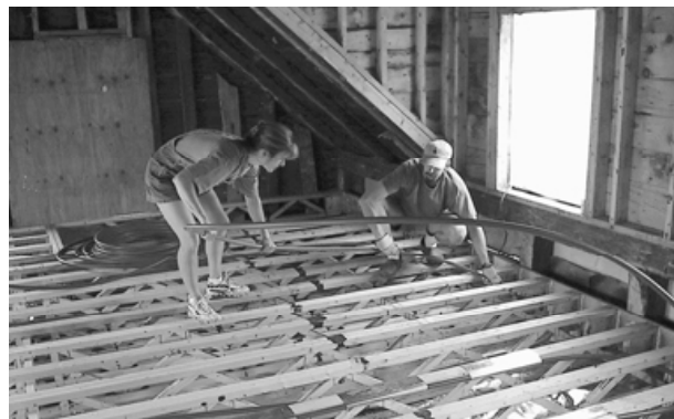
Trusses are so wide open that running 7/8" PEX through the bays becomes a very simple job.
