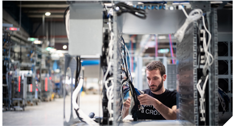
OVHcloud employee building a rack
