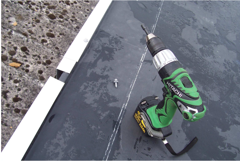
The photograph above illustrates an internal butt joint on the fascia edge
