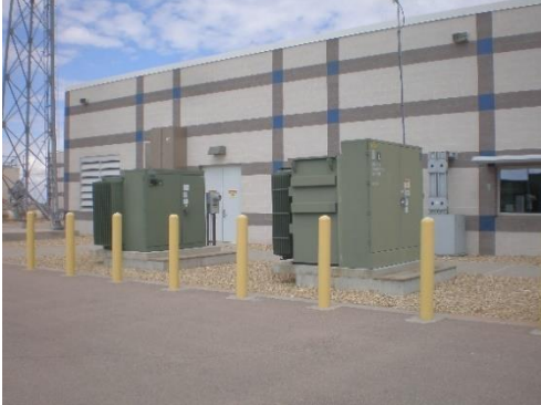
Figure 23 – The transformers that power the KBH desalination plant (Photo Credit: Art Ruiz)
