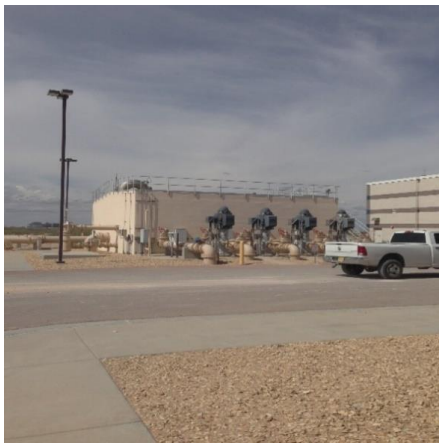
Figure 31 – Permeate pumps that lead freshwater to EPW's distribution system (Photo Credit: William Delgado-Thompson)
