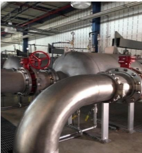
Figure 24 – Feed water pre-treatment facility (Photo Credit: William Delgado-Thompson)
