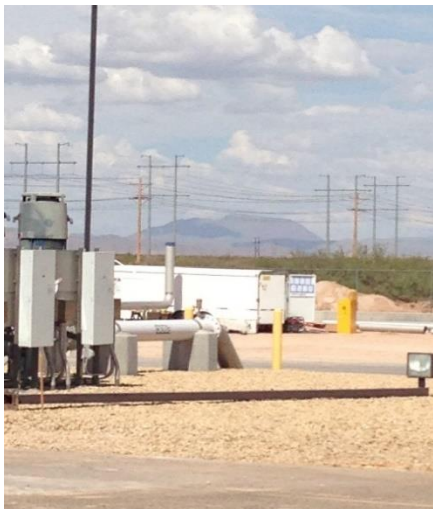
Figure 32 – Pipes that take concentrate to the injection wells (Photo Credit: William Delgado-Thompson)
