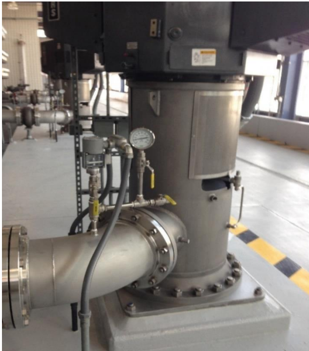
Figure 25 – High pressure feed pump that sends brackish water to membranes (Photo Credit: William Delgado-Thompson)
